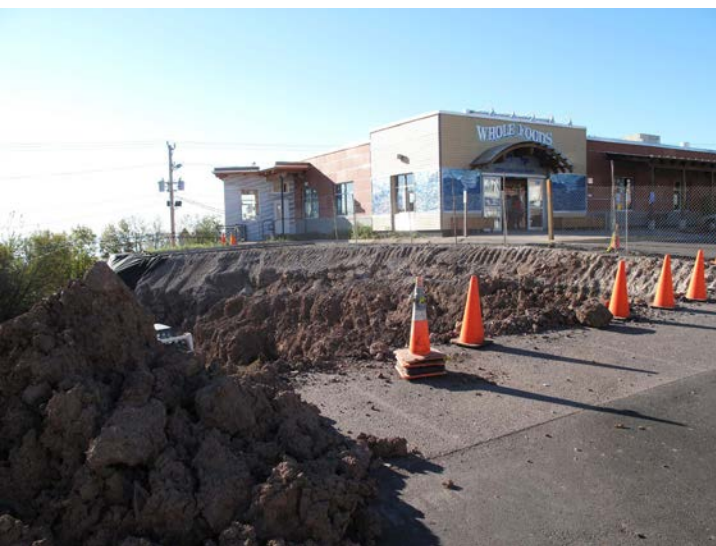
The “Great Flood of 2012,” destroyed a portion of the parking lot at the Whole Foods Co-op Hillside store.
